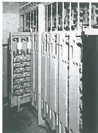
Rectifier tray withdrawn for inspection
