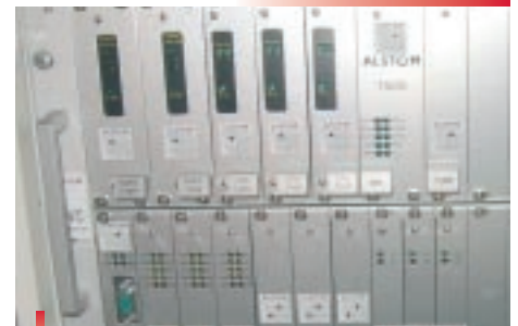
The TASS computer is vital to train operation – it is triple redundant with a two-out-of-three voting system to ensure safe operation in tilt.
