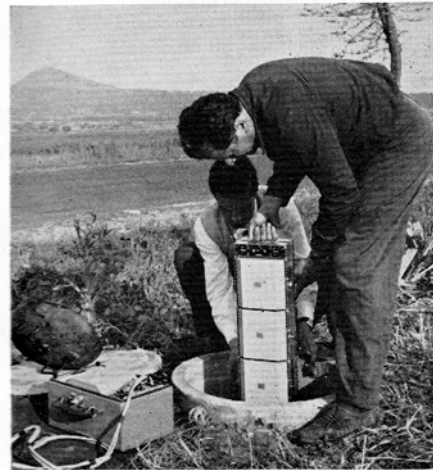
Installing STC 300-circuit trunk telephone system in Sardinia
