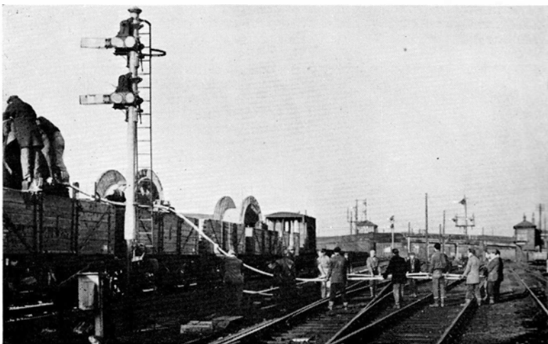
Pulling AEI 25 kV concentric oil-filled cable off cable train between Motherwell and Sunnyside for Glasgow Suburban electrification
