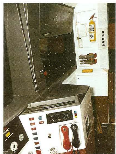
Inside view of driving cab
